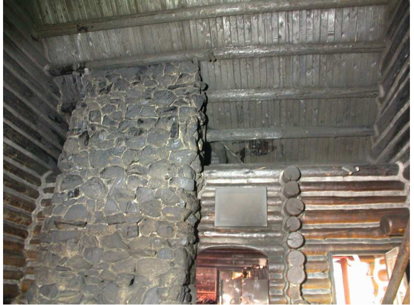
Above: Home structurally intact after fire.
